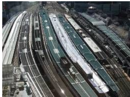
Solar Power Generation Panels
